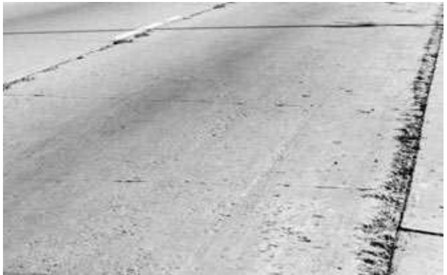
▶ Spalling along longitudinal joints.
