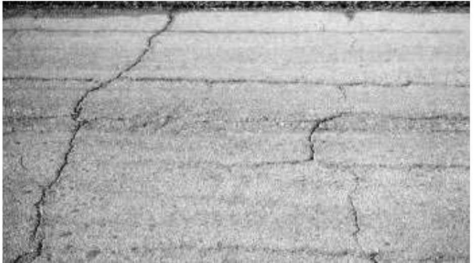
▼ Block cracking with open cracks.
