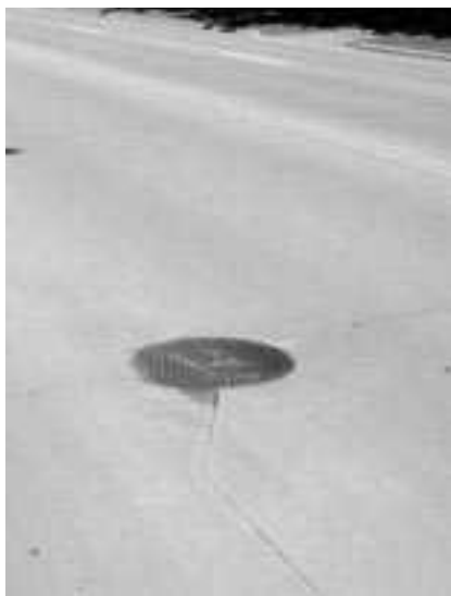
▶ Isolated spall at manhole.
