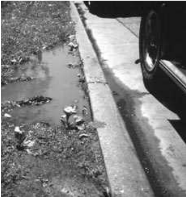
▲ Reshape terrace behind curb to restore drainage and prevent damage to curb and street.
