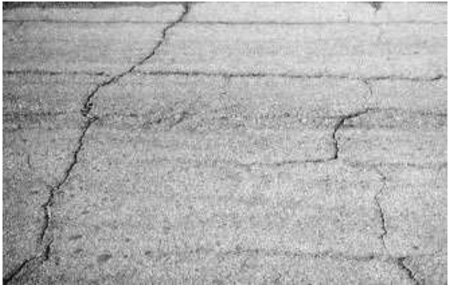
▶ Intermediate-size block cracking, 1'-5' across with open cracks.
