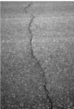
▲ Tight cracks less than 1/4" in width.
