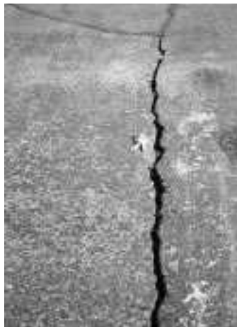
▲ Open crack – 1/2" or more in width.
