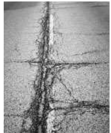
▲ Pavement ravels and erodes along open cracks causing deterioration.
