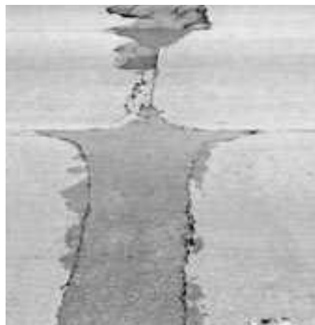
▲ Asphalt patches. Poor (top) and fair (bottom) condition.
