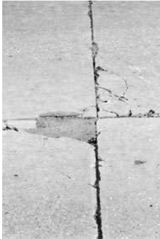
▶ Broken corner pieces. Some joint spalling.
