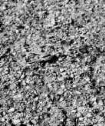
Severe raveling with ▼ extreme loss of aggregate.
