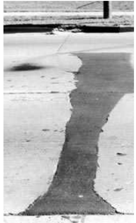
▼ Patching in fair condition.
