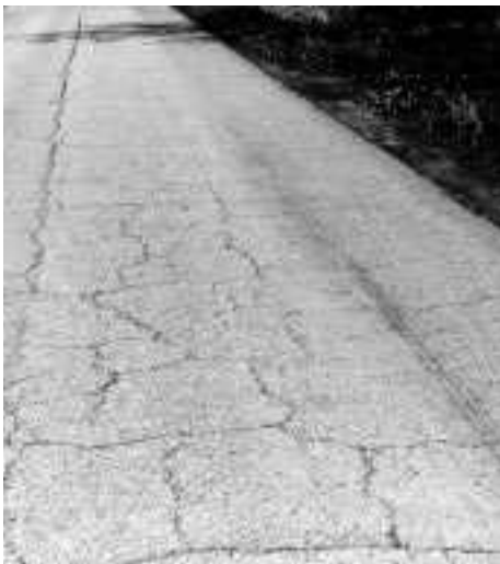
▲ Extensive block cracking in an irregular pattern.
