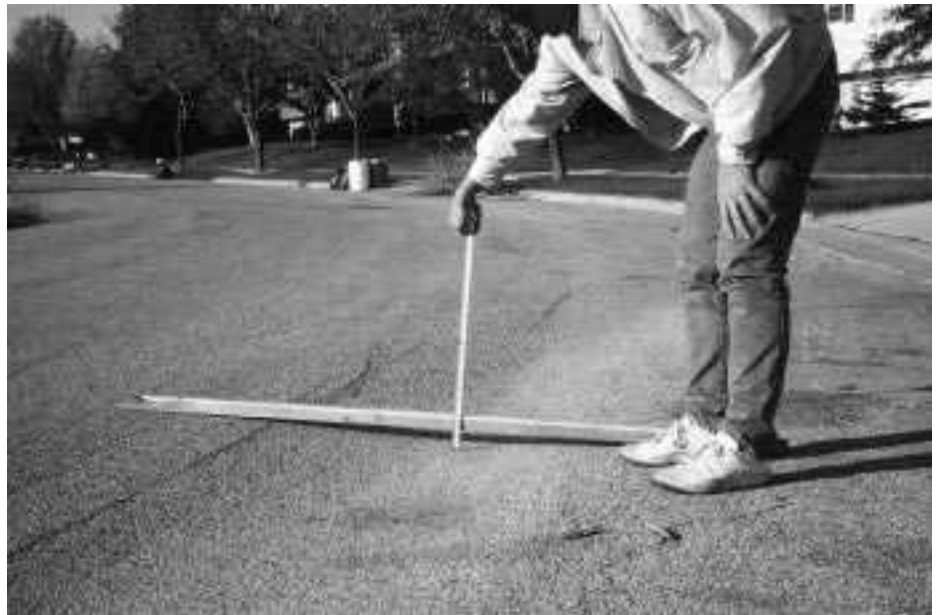
► Severe settling from utility trench.
