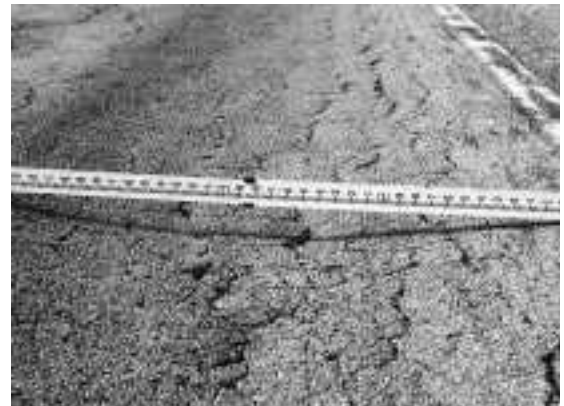
▲ Severe rutting. Strengthen base and reconstruct.
