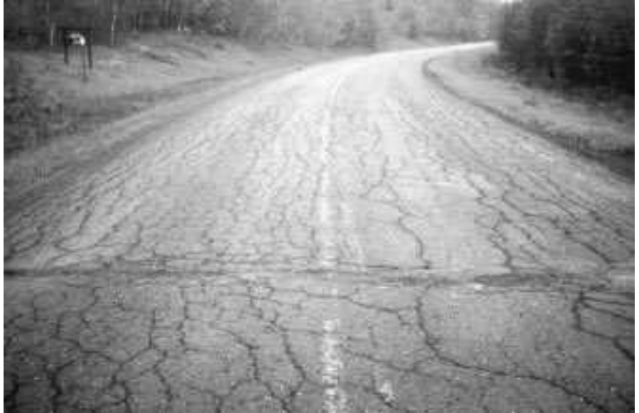
▶ Extensive alligator cracking. Pulverize and rebuild.
