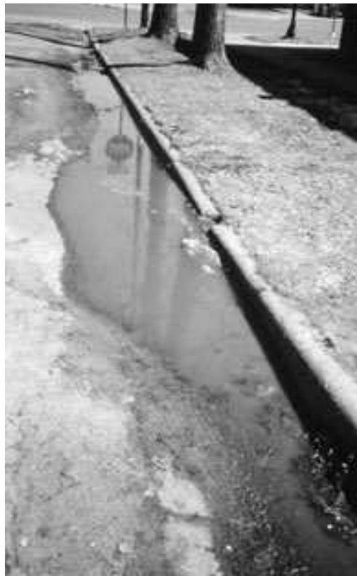
► Flooding. Curb and gutter need reconstruction.
