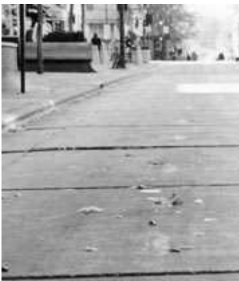
▲ Minor faulting of transverse joints. Aggravated by heavy traffic. Surface grinding will improve ride.
