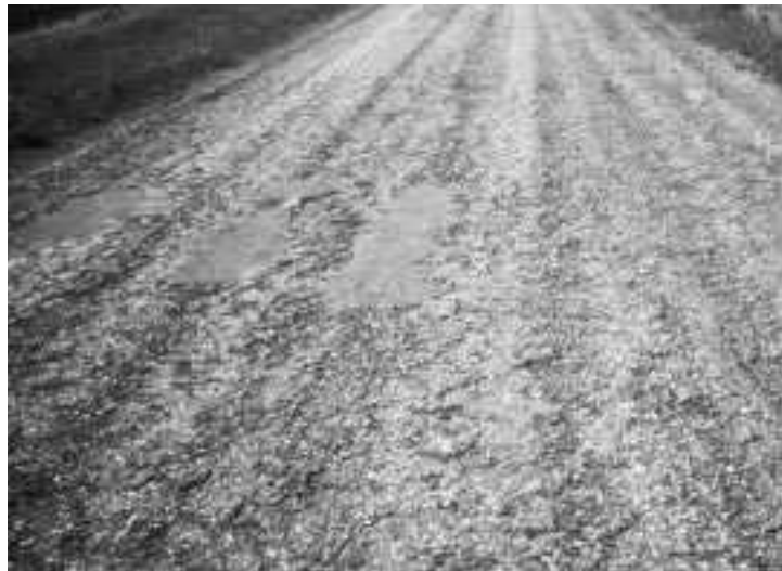
◀ Severe raveling and loss of surface material.
