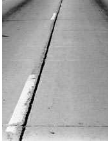
▲ Joint open about 1/2".
