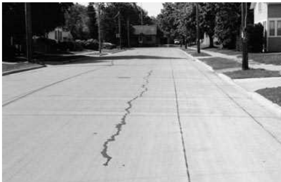
▶ Isolated meander crack, tight and well sealed.
