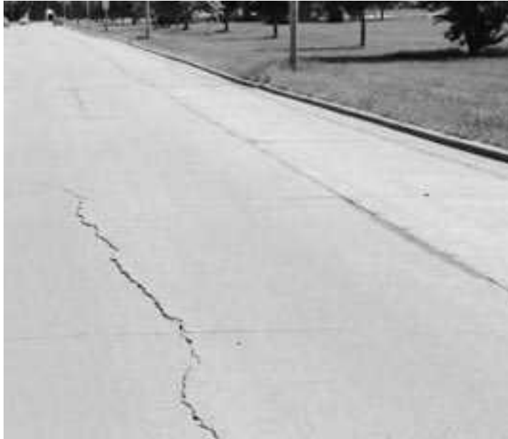
► Settlement caused meander crack with faulting.
