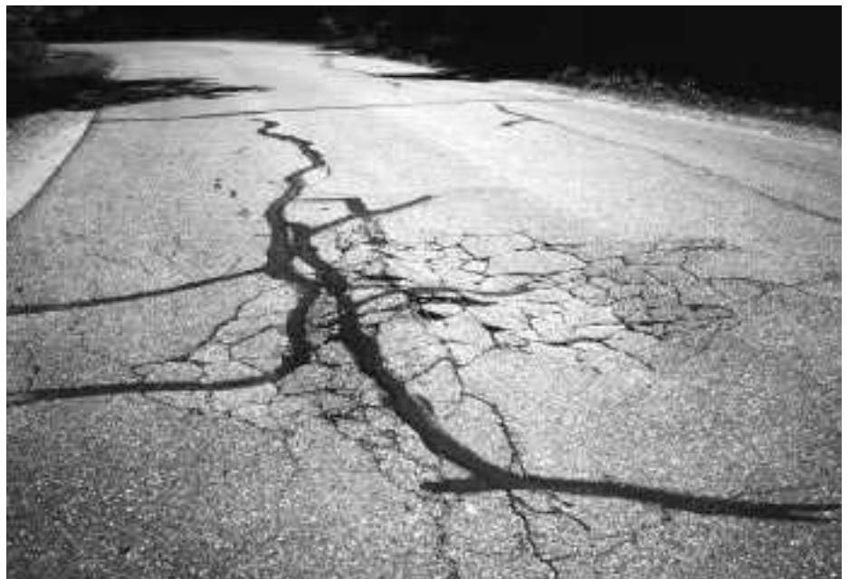
► Frost heave damage from spring break-up.
