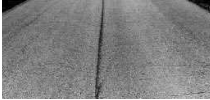
Centerline crack (still tight). ▶
