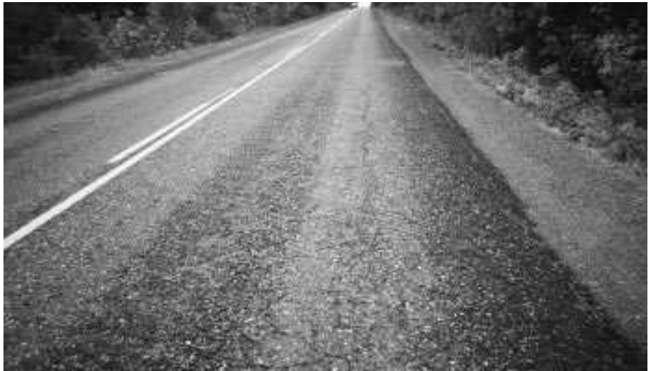
► Moderate to severe raveling in wheel paths.
