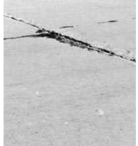
▼ Transverse joint has slight faulting and spalling.
