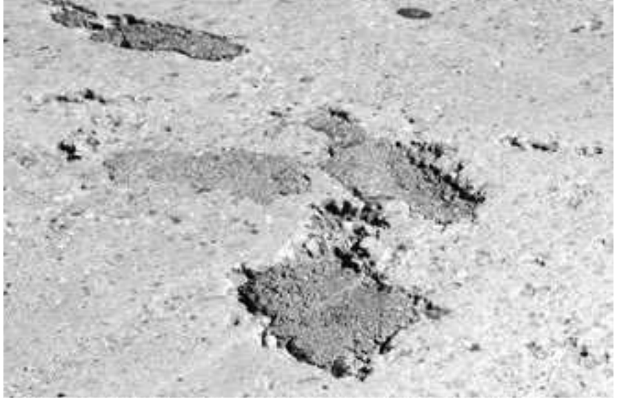
▶ Small surface spalls that have been patched.
