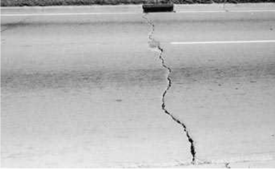
◀ Transverse, open crack.
