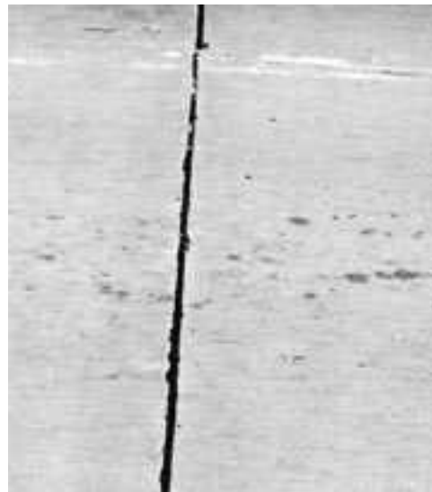
▲ Partial loss of joint sealant.
