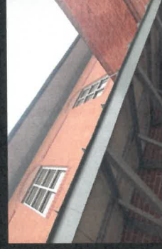
Gutters Unknown Custom Fab
